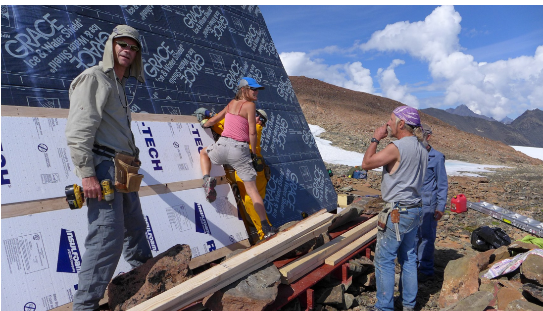
Ross Noffsinger, Sally Balchin, Stan Olsen, and Tom Choate (left to right) insulating Hans' Hut; photo by Wayne Todd
