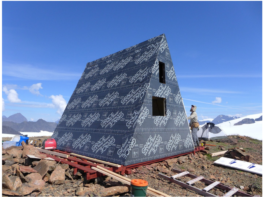
Ross Noffsinger working on the ice and water shield; photo by Wayne Todd
