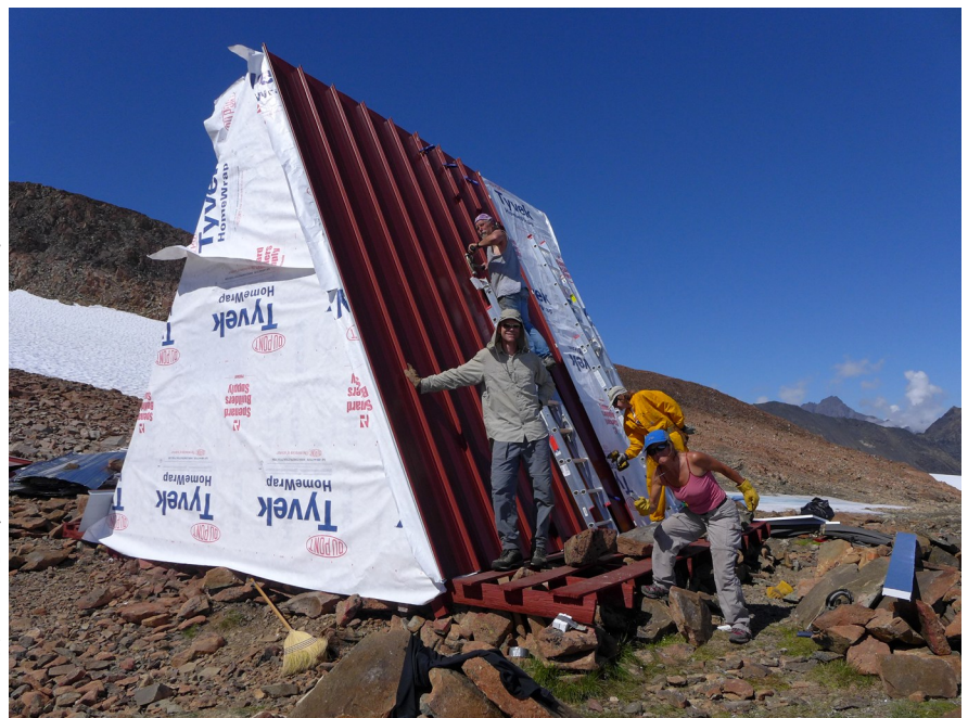
Stan Olsen (on ladder), Ross Noffsinger, Vicky Lytle, and Sally Balchin (bottom) installing metal; photo by Wayne Todd
