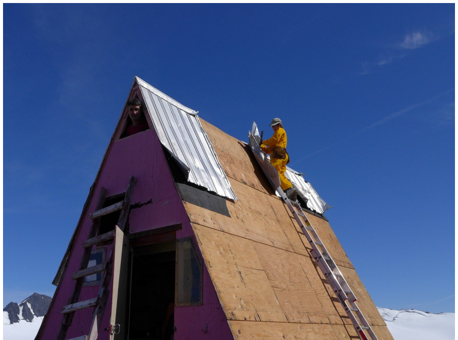
Larry Oliver peers out of the hut as Vicky Lytle conducts the tear off; photo by Wayne Todd.
