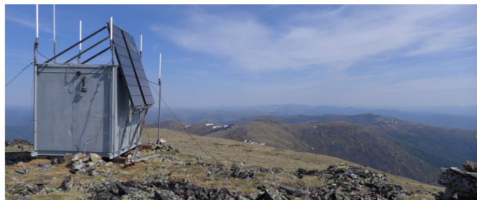
Communications shed on the summit of Chena Dome. Photo by Wayne Todd.
