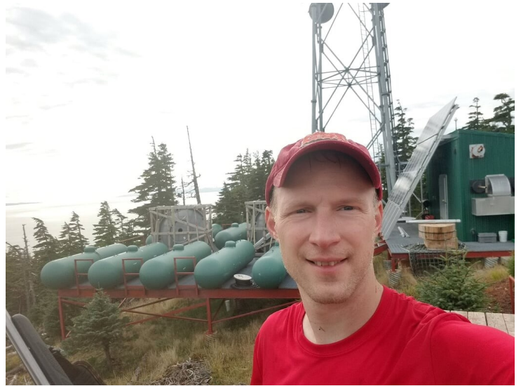
Lee Helzer in front of the generator power for the mega communications site near the Naked Island highpoint.
